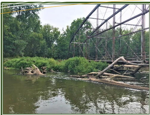
Major obstruction at State Line Bridge in Lake Village, IN (September 2019)
