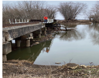
Debris at railroad bridge (Upstream)
