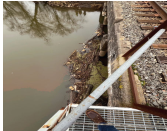
Debris beginning to show potential blockage (Upstream)
