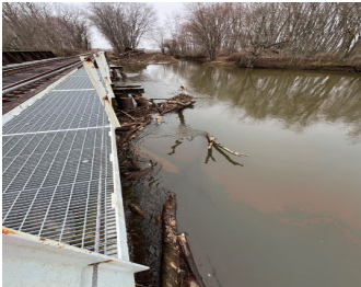
Debris beginning to show blockage (Upstream)
