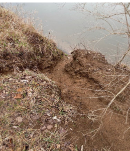
Breach area forming
