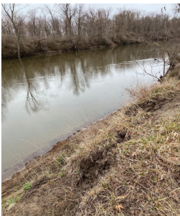
Tear in side, bank sluffing into the river
