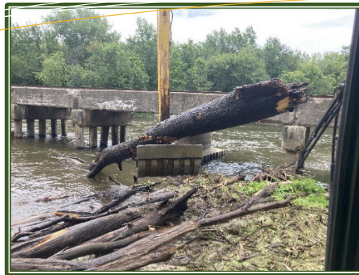
Workers remove a logjam from an over century-old bridge over the Kankakee River (July 2024).
